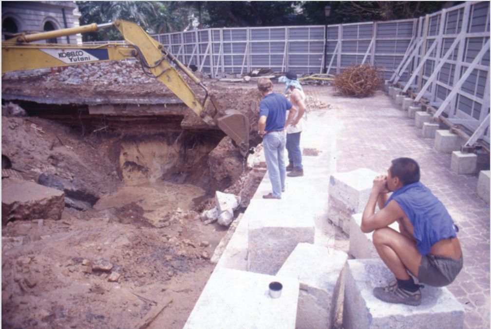
5.32 Omar Chen and Mike Flecker viewing the EMP construction site, January 1998. A thick black sand layer seemed to offer good potential, but archaeologists were not permitted to enter the pit to take samples of the soil or artifacts due to safety considerations.
