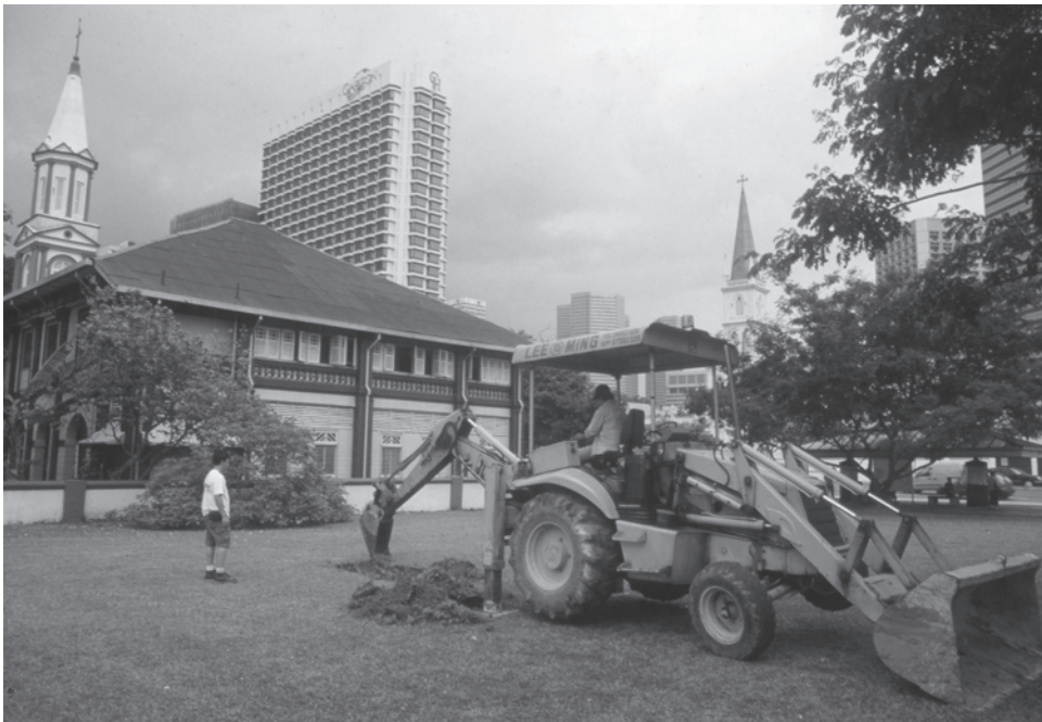
5.01. Bras Basah Park, now the site of the Singapore Management University, during the test excavation with backhoe
