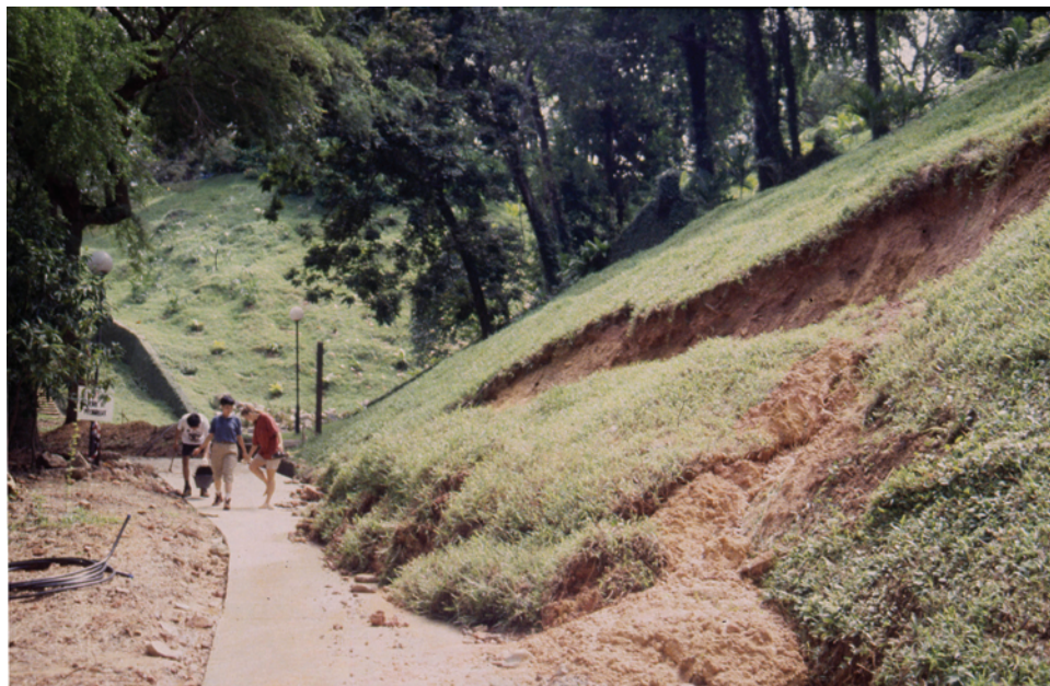
5.22 Landslide on River Valley Road slope of Fort Canning
