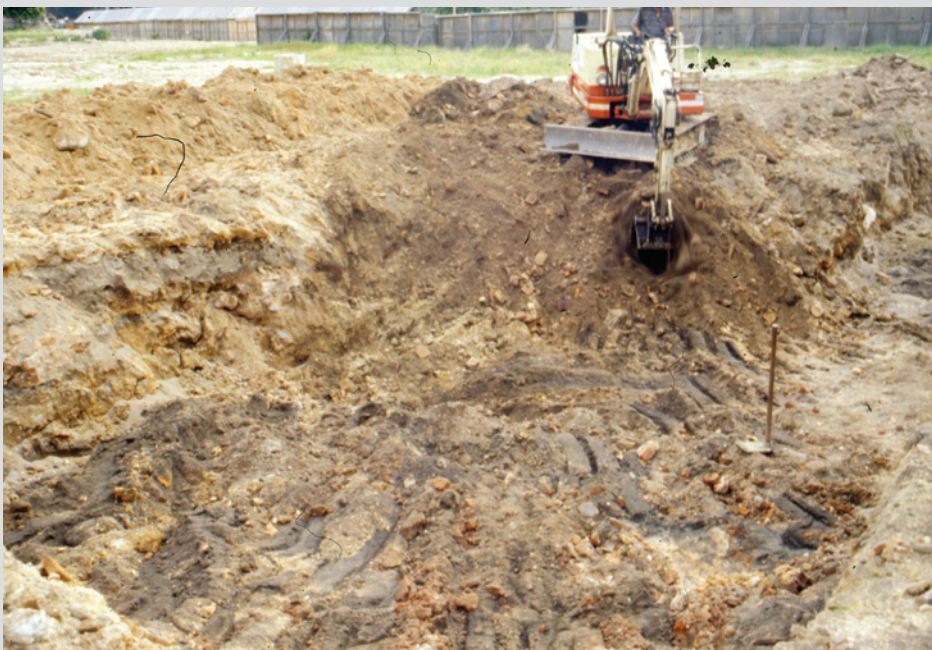
5.29 Backhoe clearing topsoil from the fourteenth-century layer at Parliament House Complex. The layer of black sand containing fourteenth-century remains is just beginning to appear.
