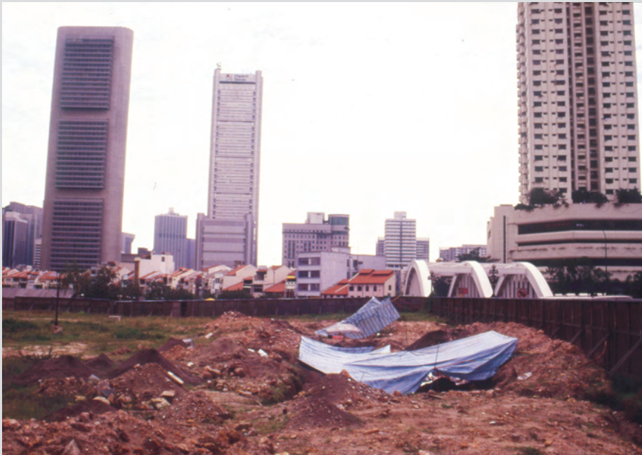
5.28 Parliament House Complex excavation, sheltered by blue and white striped sheets. This picture was taken from the corner of North Bridge Road and High Street, looking toward the Singapore River.
