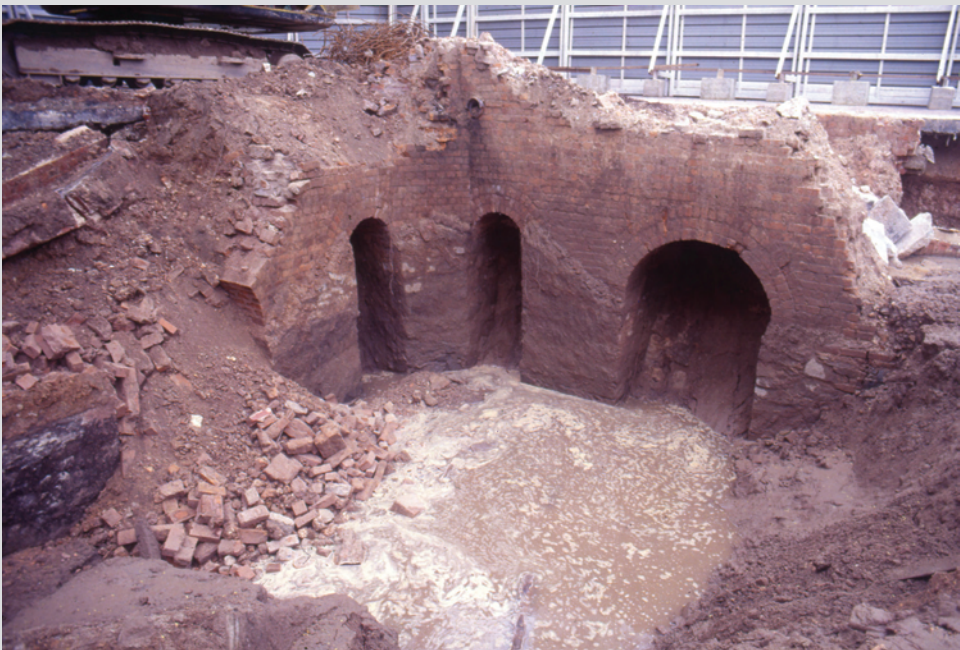
5.37 Demolition of the nineteenth-century treasury at Empress Place, beneath the former hawker centre
