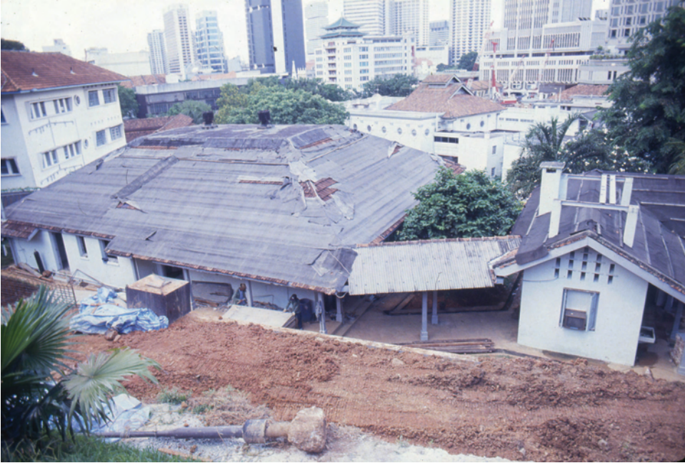
5.20 The Fire Director's Residence behind the Hill Street Fire Station during renovation
